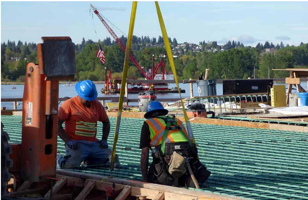
WABN crew members install rebar for the final section of the new WABN roadway deck.
